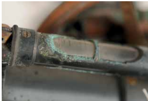
Figure 6. Glass levelling gauge causing corrosion on the mounting brass. Photo: M. Braun.
